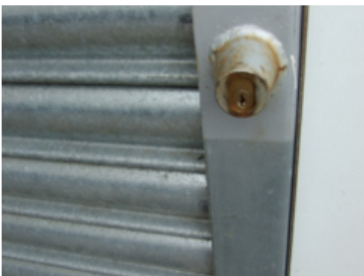
Locking barrel returned without key – needs to be drilled and replaced
