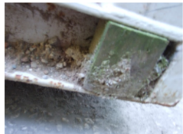
Concrete splashes on base of unit
