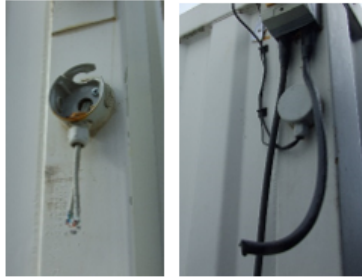
Damage to Wiskq box and damage to electrics
