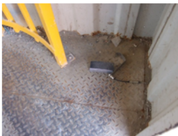
Dirt, rubble and rubbish left in unit to be tidied and cleaned
