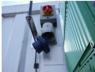
Damaged Commando Socket
