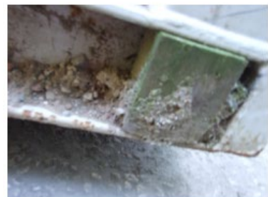
Concrete splashes on base of unit
