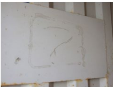
Glue and adhesive remaining on internal walls and panels
