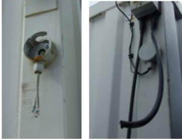
Damage to Wisk box and damage to electrics
