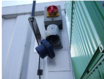
Damaged Commando Socket
